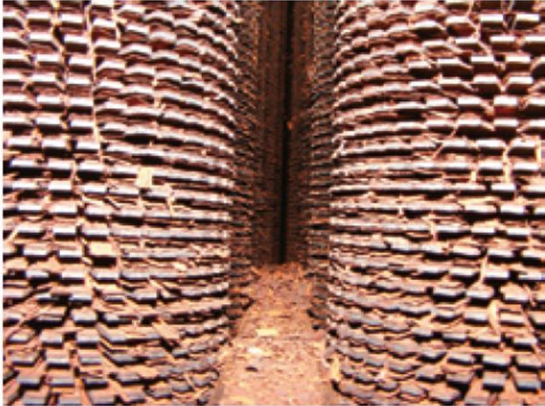
5. Tube bundle is fouled with rust and other deposits
