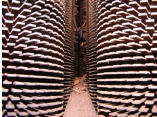
6. First cleaning pass using CO 2 eliminates most deposition on tubes near the face of the tube bundle
