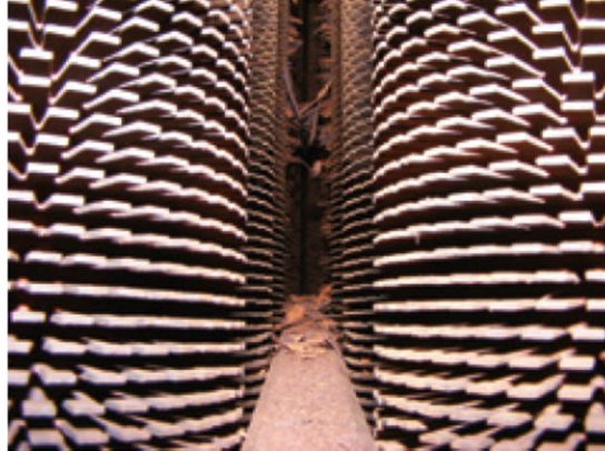
6. First cleaning pass using CO 2 eliminates most deposition on tubes near the face of the tube bundle
