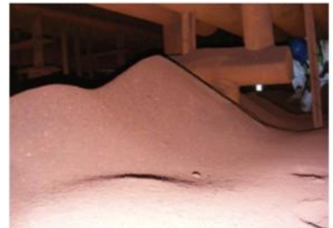
9. Foreign material removed from finned tubes must be collected and sent to a landfill
